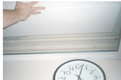
^ ORIGINAL WOOD TRIM ABOVE THE CEILING TILES.
