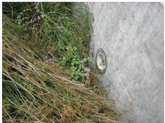
Figure 8: Filtration Planter 4 Outfall from Roof
