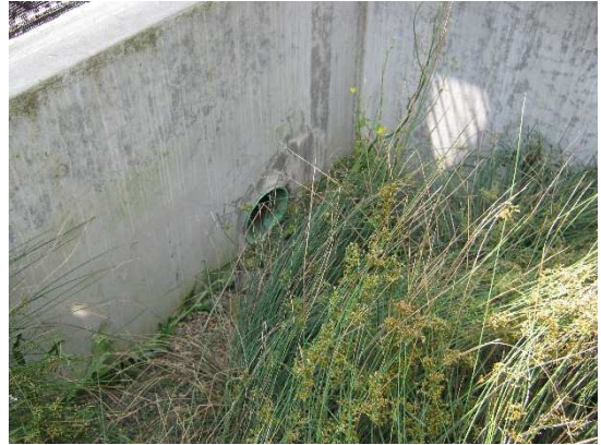
Figure 6: Filtration Planter 3 Outfall
