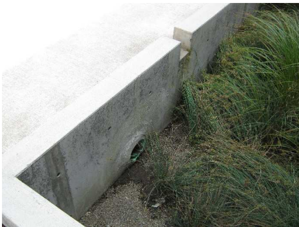
Figure 4: Filtration Planter 2 Outfall
