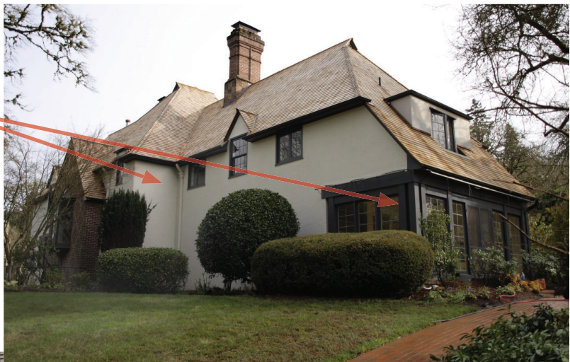
2009 - North/West facade showing circular window missing and living porch is enclosed (date unknown).
