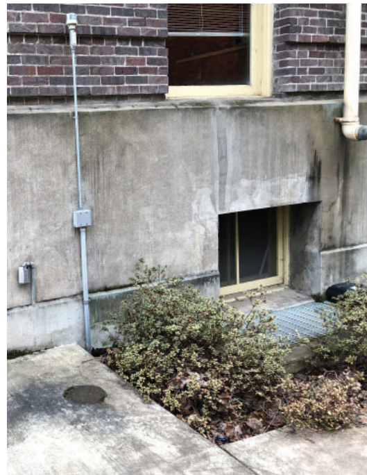
Foundation showing repairs, mechanical equipment added to facade is not original.
