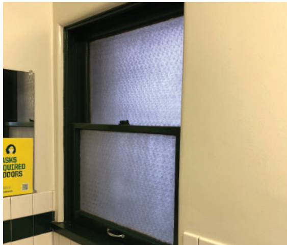
Room 207 Womens Restroom
