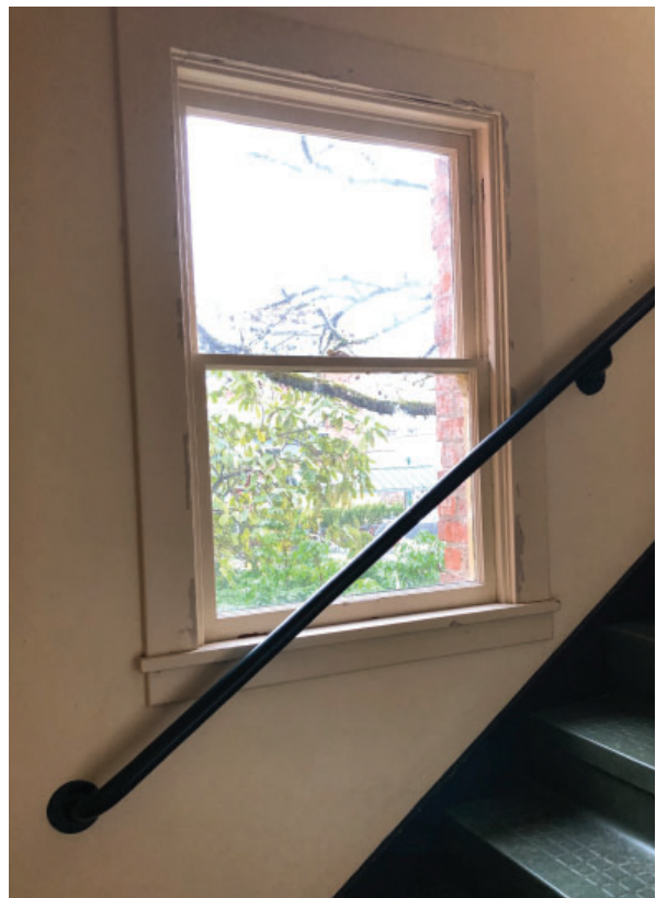
First Floor Stairwell (Railing intersects window)
