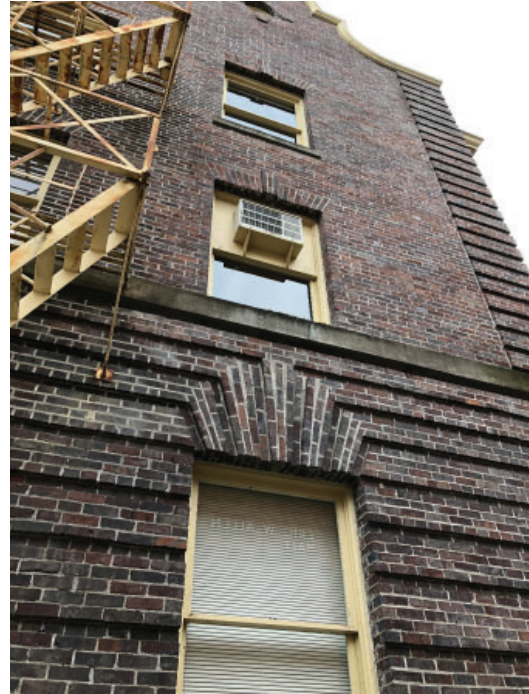
AC units installed in windows, not original.
