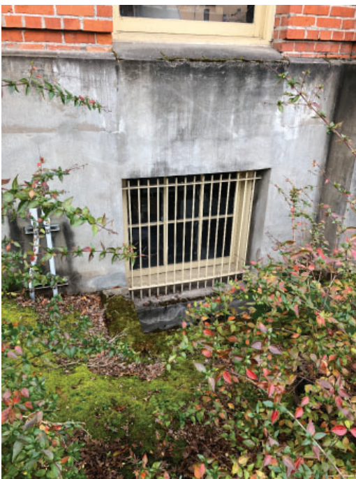
Water damage on window sills; basement windows with bars that are not original.
