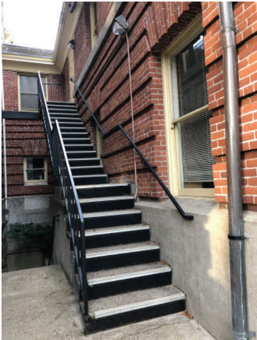
Light fixtures are not original. Foundation differences between basement and ground level.
