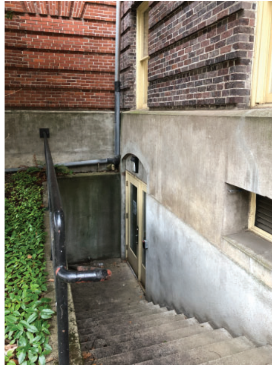
Stairwell leading down to basement shows foundation differences. Brick color differences between additions and original building.
