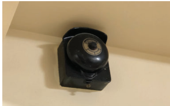
Third Floor Hallway (Old Fire Alarm)
