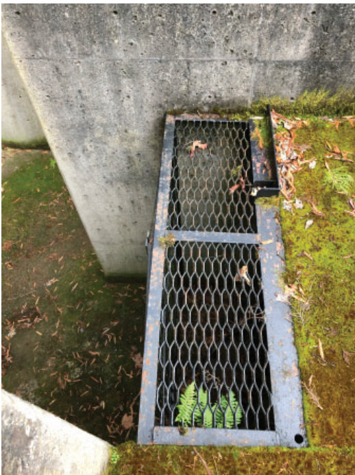
Original accessibility lift is currently not operable and not original.
