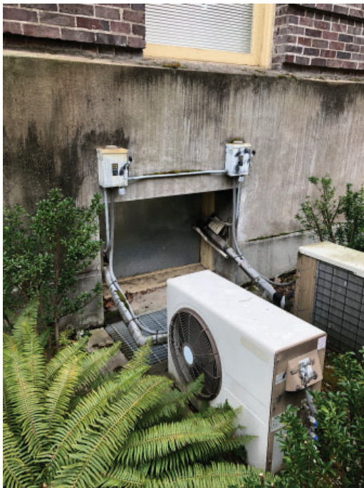
Mechanical equipment added to exterior with exposed connections.
