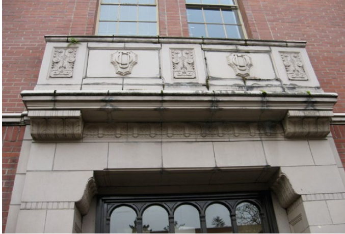
Terracotta detailing consistent with original drawings. Indicates that the original vestibule likely had terracotta detailing as shown on drawing (see p. 25 and 27). 2011.
