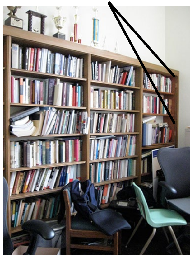
Original built-in bookcases in Room 222. Notice the missing cabinet doors in the far right. March 2015.
