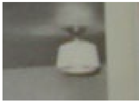
Original ceiling mounted lighting fixture. 1945.
