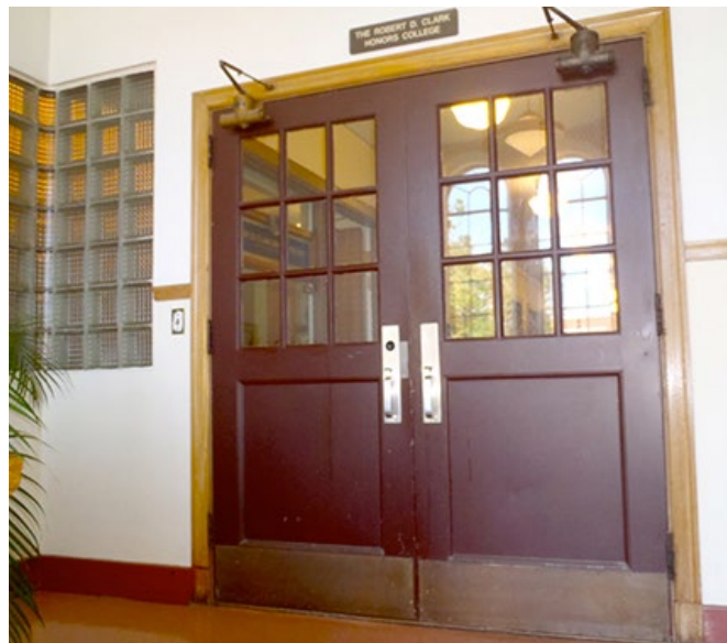
Entry to third floor from main stairwell showing double doors and glass block. 2011.
