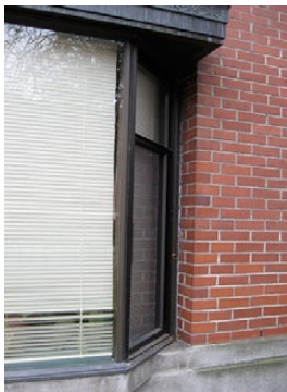
Operable window unit installed in west portion of bay window. 2011.
