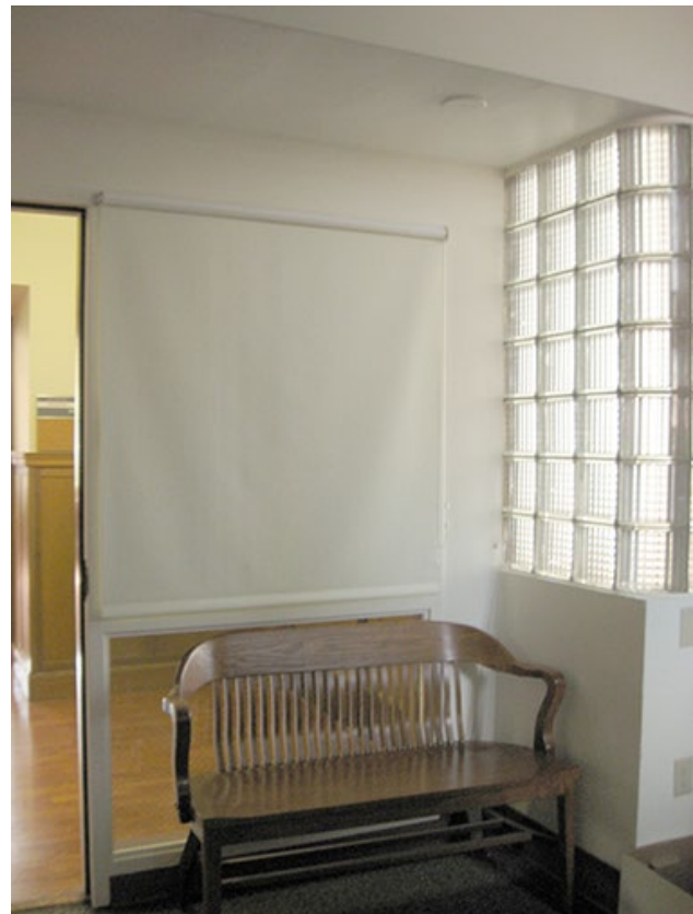
Room 320 looking south. Note original glass block. Originally a built-in counter stood where the storefront window system and bench is located in the photo. March 2015.
