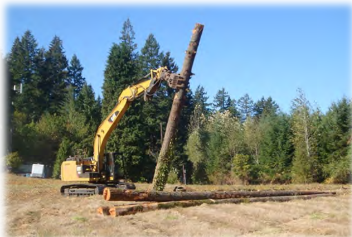
Habitat snag being installed in an area with no mature trees (Source: Metro)
