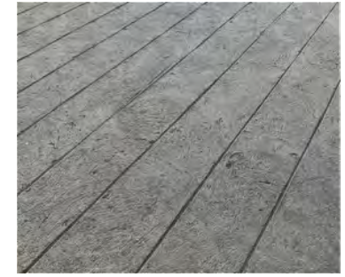
5: Cast in place concrete - Grooved finish with dark color Indicates transition to mixing zones
