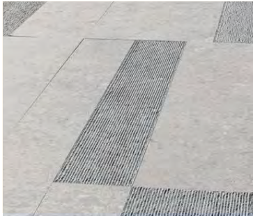
1: Cast in place concrete - Varied texture finish Pedestrian scale paving pattern Color change in wheels zone
