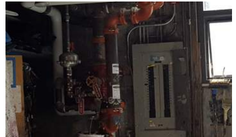
Fire water service entering the building
