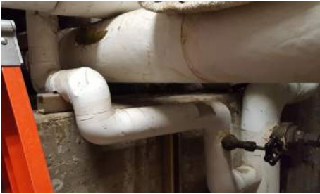
Chilled Water and Steam entering the building from the tunnel system
