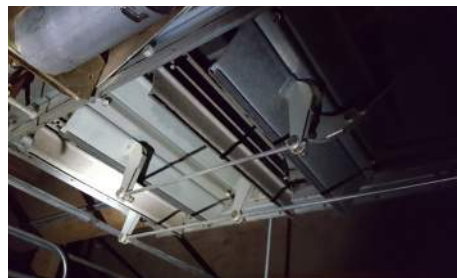
Typical Roof Relief Damper
