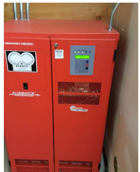
New emergency lighting inverter system provided as part of the 2009 renovation
