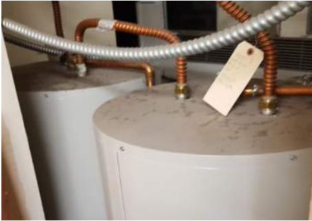
Electric Hot Water Heaters in Villard Hall
