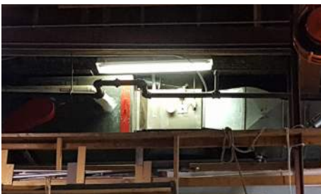
Minor Theater Air Handling Unit
