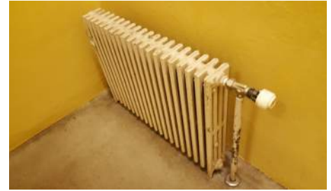
Existing cast iron steam radiator
