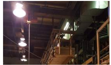
Existing Metal Halide and Fluorescent fixtures used at Theater backstage area
