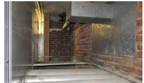
Main service conduits coming into main gear
