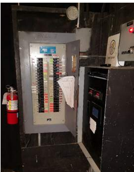
Existing Panel "I" (above) and Panel "J" (below) serving backstage lights, receptacle cord/reel, paint shop, and receptacles above the theater.
