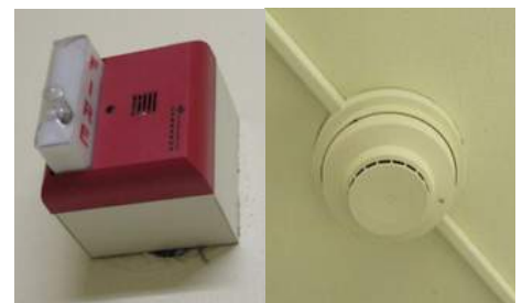
Typical fire alarm devices in building
