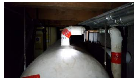
Asbestos Covered Equipment
