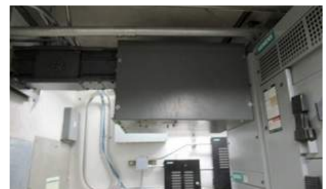
Working clearance issues in main electrical room (Bus-riser pictured)
