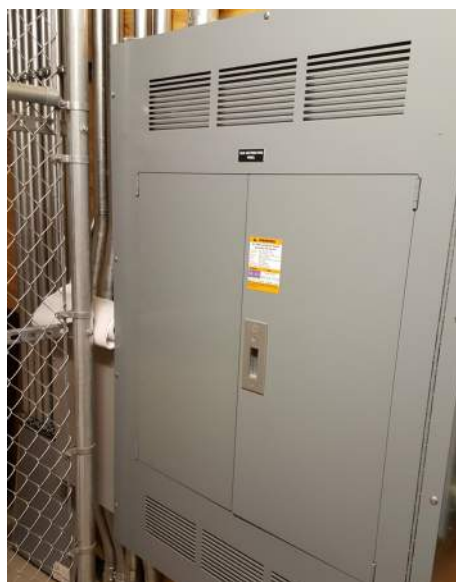
New 800A 208/120V, 3-phase, 4-wire sub-distribution panel serving the theater addition
