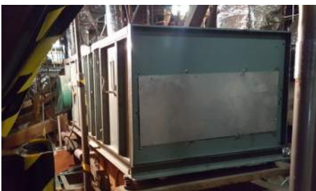
Abandoned AHU in Villard Hall Attic
