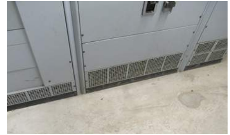
Main gear not located on a raised equipment pad and no seismic support.
