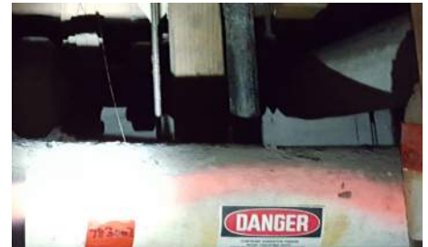
Asbestos Covered Piping
