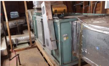
Typical AHU in Villard Hall Attic
