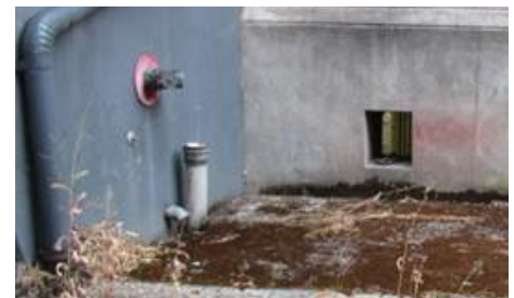
Opening into main electrical room
