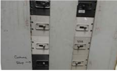
Custom made/modified distribution panelboard
