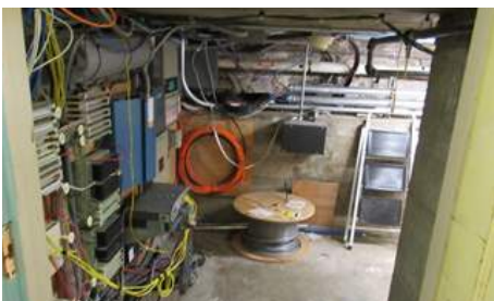
Current demark location for low voltage services
