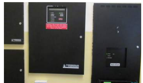
Main fire alarm control panel
