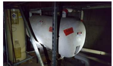
Abandoned water heater and storage tank.
