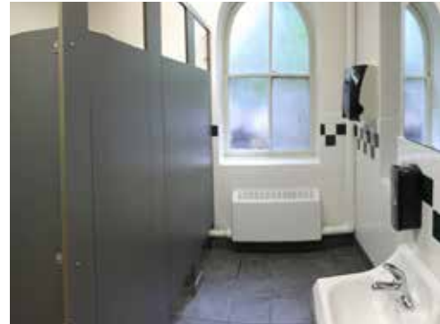
Image 53: A typical restroom adjacent to the interior stairs at the southeast or southwest corner of the building. No ADA stalls exist at these locations.
