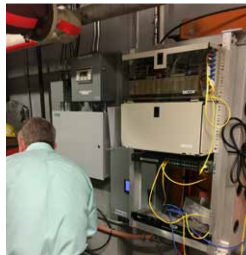
IMAGE E3: Campus fiber optics rack in boiler room.
