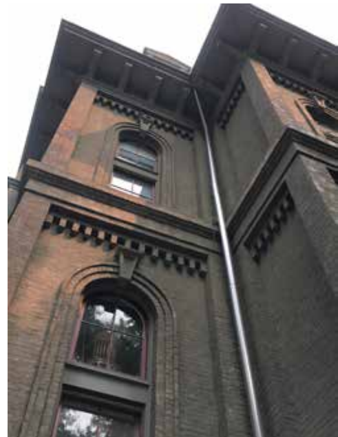
Image 8: Detail of exterior masonry features that include brick pilasters, belt courses with dentils, and rowlock arches.
