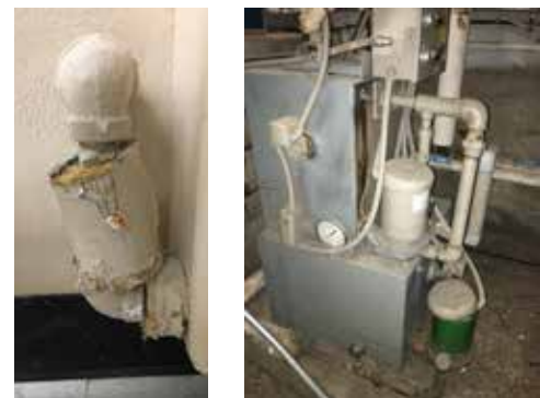
IMAGE M3: Heating system piping and equipment in disrepair.
