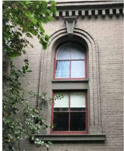
Image 23: One of six windows converted to pivoting sash with a broad horizontal mullion. These date to 1914 when the floor levels were subdivided with the introduction of mezzanines.
