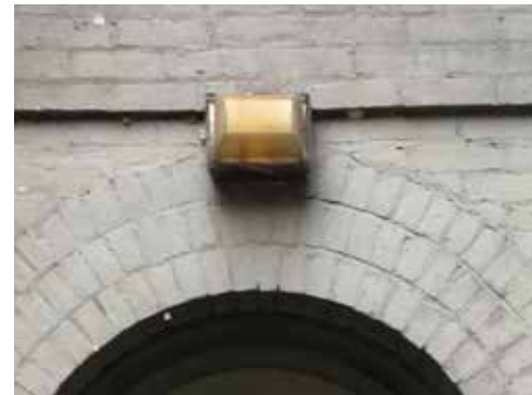
Image 36: A typical exterior security sconce used at entrances.
