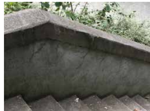
Image 18: Cracking and spalling along the concrete cap of the exterior stair wing walls, and continuous hairline cracking.
