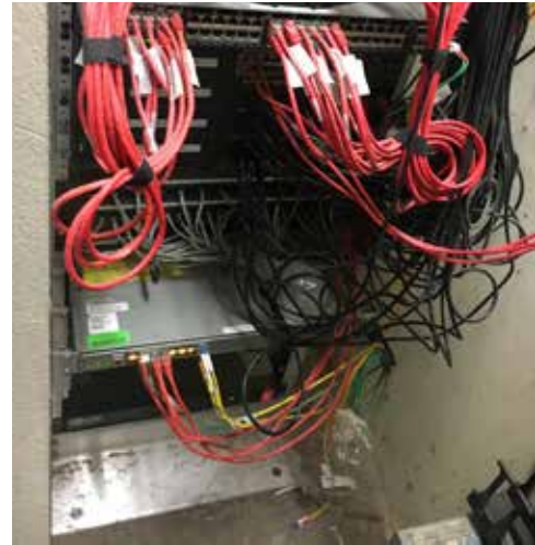
IMAGE E4: Servers and Cat 5e cabling chase space next to elevator in basement.
