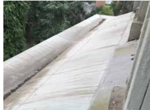
Image 20: Detail of the roof membrane at the third floor dormers. Although stained, the membrane appears intact.
