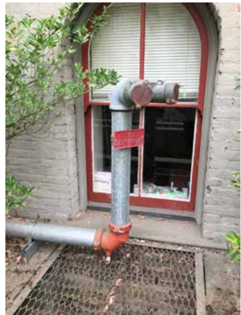
IMAGE FP2: Exterior fire department connection along the north elevation.
