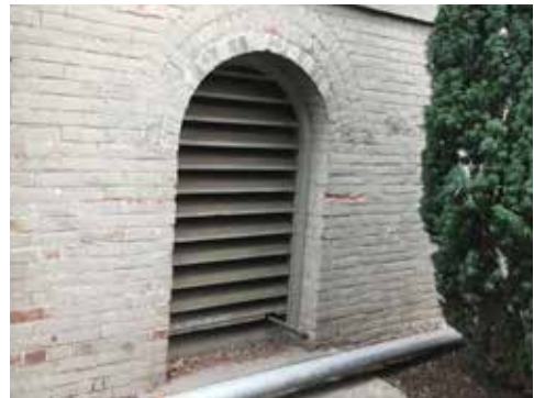
Image 24: One of two louvered window openings at the basement elevation. Original wood sash are believed to be held by UO in storage.
