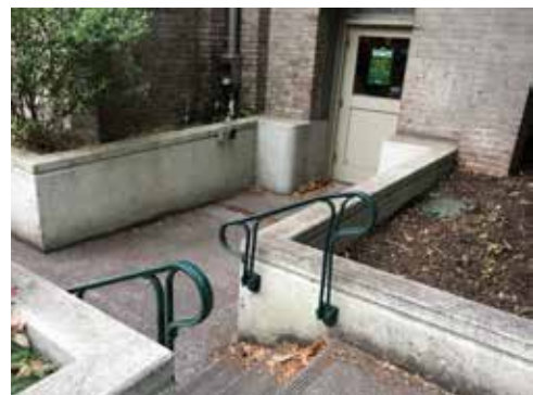
Image 45: Detail of the ADA entrance at the northwest corner of the building. This basement entrance is accessed by both stairs and a compliant ramp.
