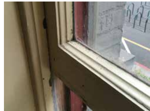
Image 27: Detail of sash bottom rail, interior ogee profile, and single pane glass. Sash thickness is substantial and could accommodate insulated panes.
