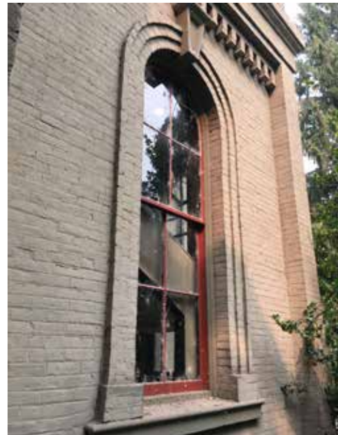
Image 3: A typical double-hung window with rowlock brick arches and a cast metal keystone and sill.
