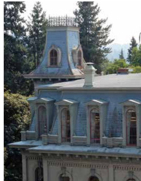
Image 19: The iconic mansard roof and tower at the east end, also mirrored at the west end. Wood shingles are weathered and the wood parapet shows signs of deterioration.
