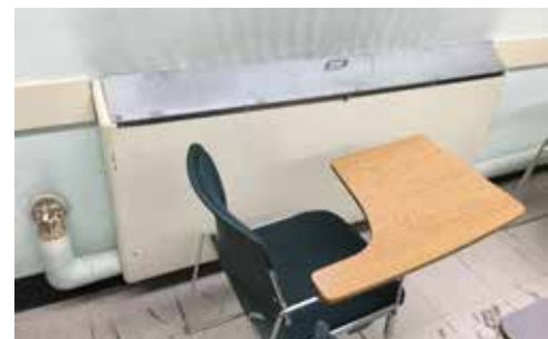
IMAGE M2: Typical radiator and cover in classroom.
