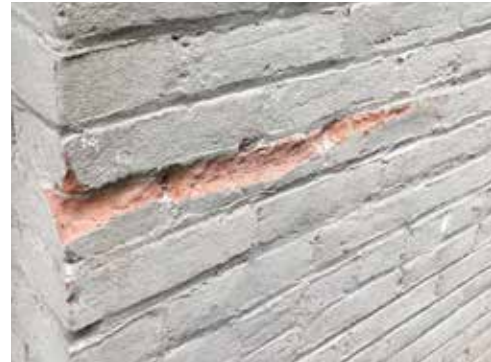
Image 14: Damaged exterior brick from an unknown external force.
