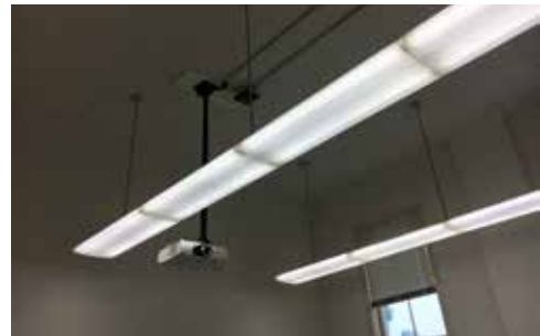
IMAGE E8: Typical fluorescent luminaires in classrooms.
