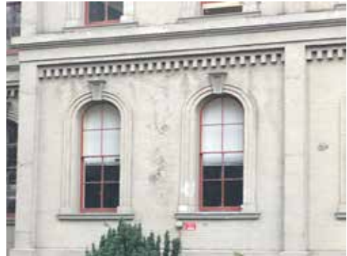
Image 11: Typical exterior soiling and staining along the north elevation.
