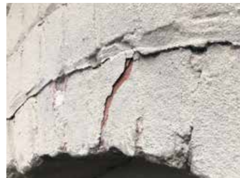
Image 10: Detail of the exterior sand painted finish coat. At areas where the coating is spalling, it is taking the brick fireskin with it.
