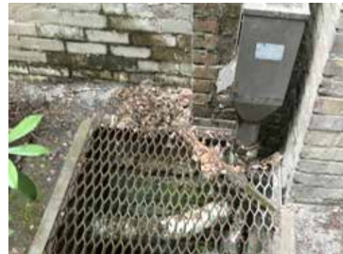
Image 74: Storm drainage and pipe access at the down spouts at each corner of the building's exterior.
