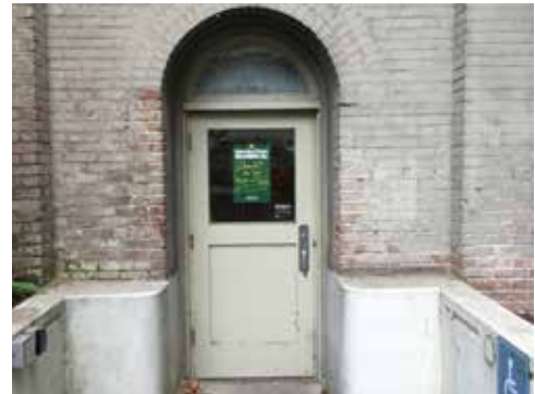
Image 30: Door slabs at the north elevation basement entrances are half-lite modern replacements. Original units were 5-panel wood doors.
