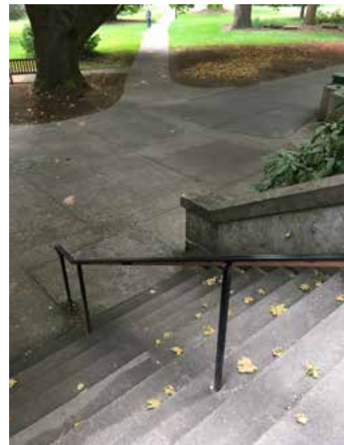
Image 16: Detail of concrete exterior stairs along the east and west elevations. Tread noses have been patched (lighter in color) and a modern metal rail runs down the center of the stair.
