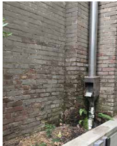
Image 13: Overspray at downspout locations causing high moisture levels along the brick exterior, deteriorating the finish coat and mortar joints and causing high levels of biogrowth.
