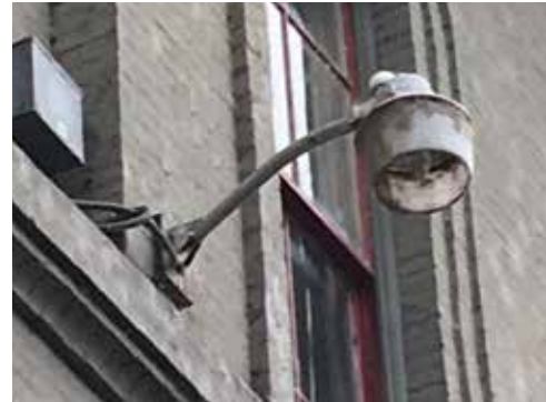
Image 35: An incompatible exterior sconce along the north elevation.
