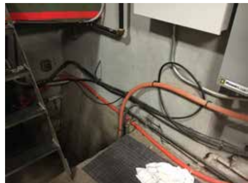
IMAGE E12: Campus fiber optics route into the building from the steam tunnel at the northeast corner at basement level.
