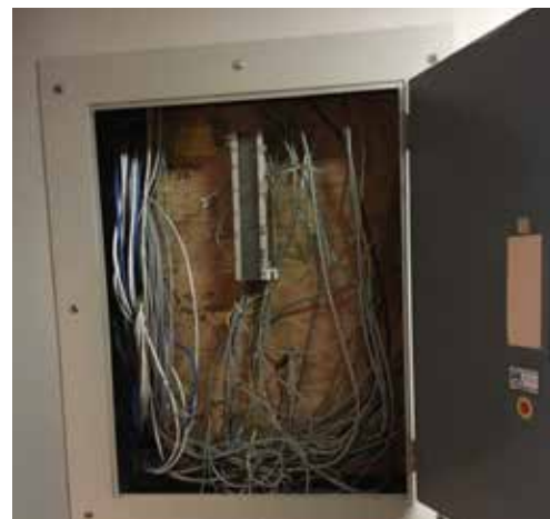
IMAGE E6: Flush-mount telephone cabinets.
