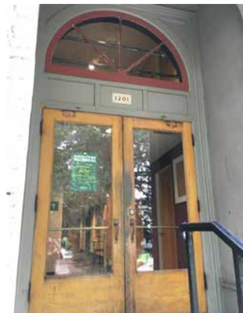
Image 28: One of two exterior double doors that serve as the main entrances centered at the east and west elevations. Door slabs are weathered at the exterior. Transom units and trim are in good painted condition.
