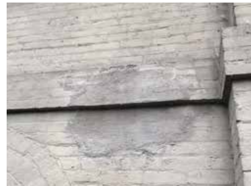
Image 15: A common cementitious infill patch, typical at the north and south elevations.
