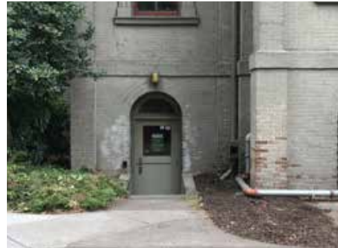
IMAGE E7: Outdoor lighting with surface raceway and boxes.
