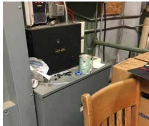
IMAGE E2: Power source terminal cabinet in the basement mechanical room.
