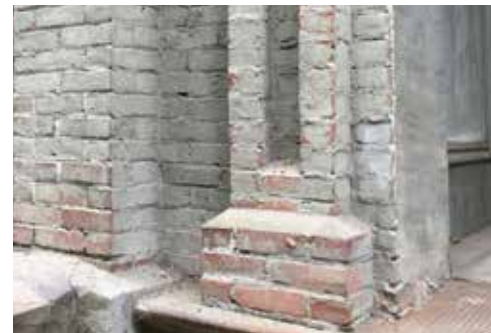
Image 9: Deteriorating exterior finish coat reveals the original red-orange brick units.
