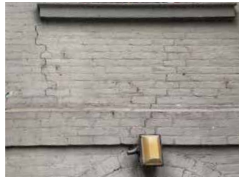
Image 12: Detail of common crack locations extending from window sills and above arched openings.
