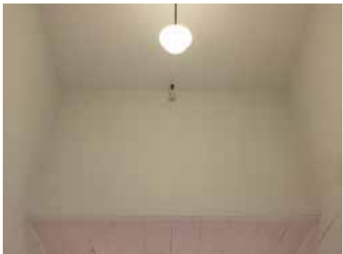
Image 25: One of two skylight shafts from 1914, currently enclosed, with pendant light fixtures.
