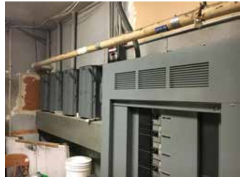
IMAGE E1: The electrical system switchboard in the basement mechanical room.
