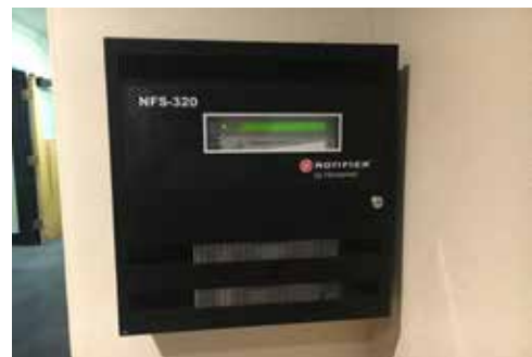
IMAGE E5: Fire alarm control panel.
