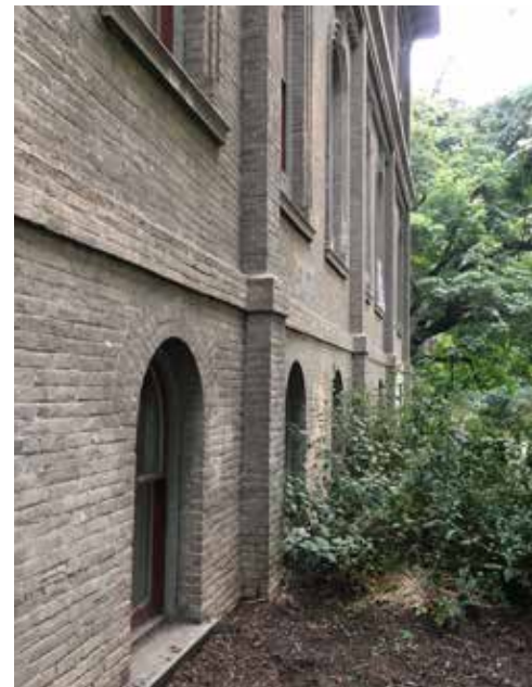
Image 37: Perimeter landscaping encroaches upon the building at all elevations.
