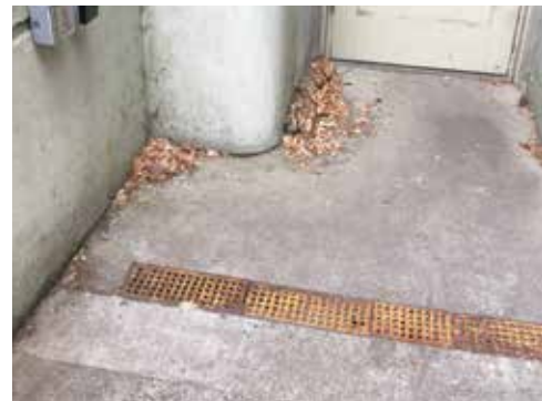
Image 75: One trench drain is located at the base of the ADA ramp at the north elevation.
