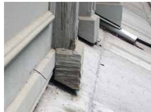
Image 21: Detail of rotting wood members hovering above the roof membrane at the wood parapet..
