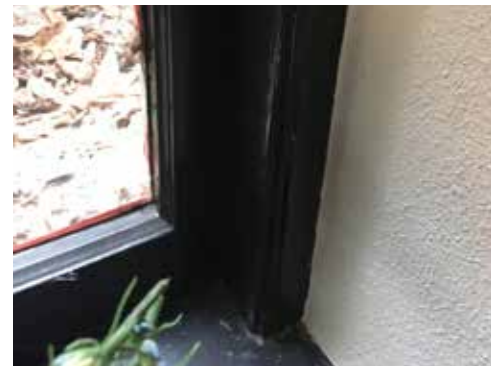
Image 69: Detail of interior window trim at a recessed window location. Recessed window trim will not be impacted by the addition of shear walls.
