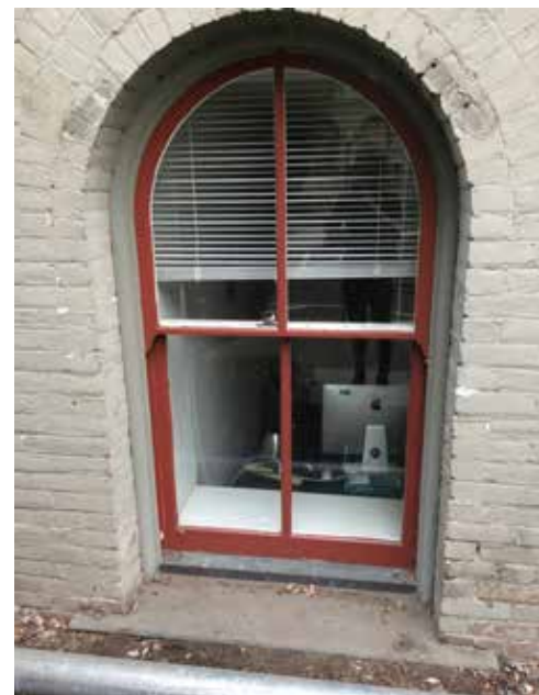
Image 22: A typical exterior double-hung window at the basement level. Units are true divided light with single panes and putty glazing. Recently restored, their painted finish is intact.
