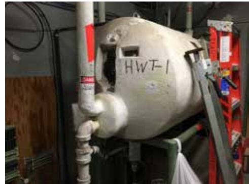
IMAGE P1: The 150-gallon storage hot water storage tank.
