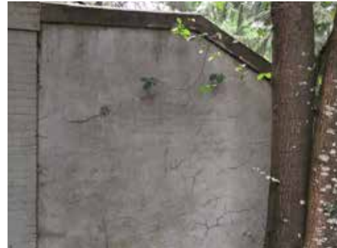
Image 17: Detail of typical hairline cracking at concrete stair wing walls.
