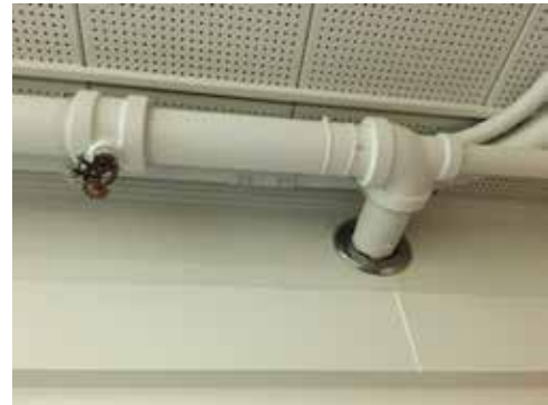
IMAGE FP1: Typical 4” fire sprinkler water line.
