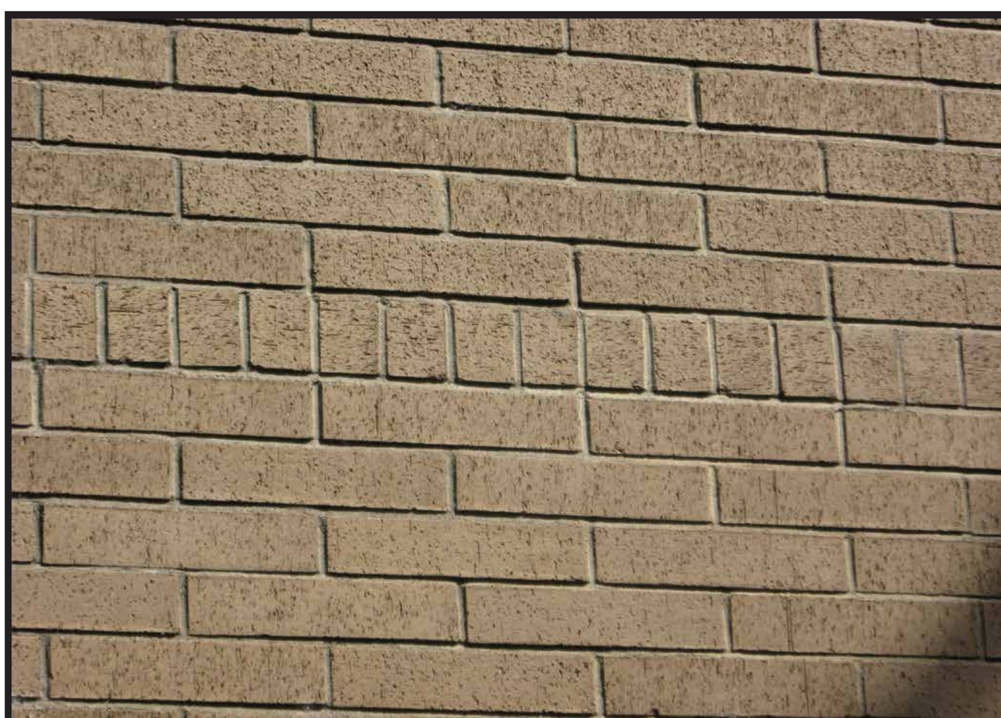
This choice of brick reflects back to the original home of the Law Department and Law Library previously housed at Fenton Hall. The yellow brick mimics the Italian Renaissance design influences of Fenton Hall. Changes in brick orientation denote floor divisions
