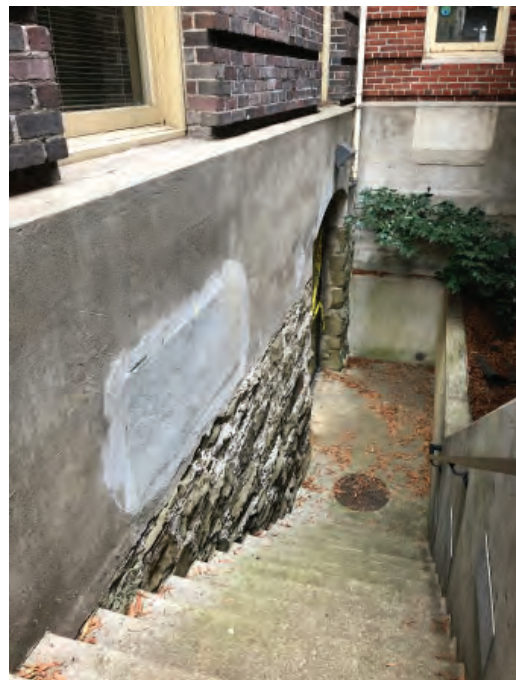
Difference between original stone foundation and 1914 addition foundation. 1914 addition used different colored brick
