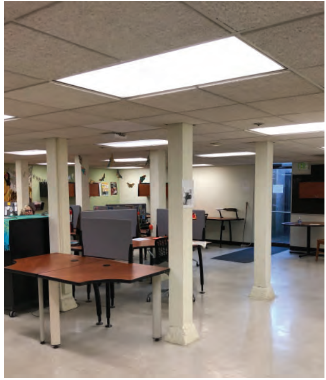
Support pillars not original; further research needed for year pillars were placed/replaced
