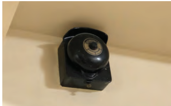
Third Floor Hallway (Old Fire Alarm)
