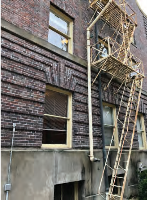
Fire escapes are not original, further research needed to determine date added. Fire sprinkler standpipes are not original.
