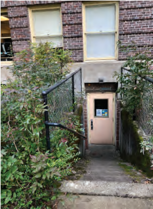
Light fixture above basement door is not original. Fenced stairwell is not original.
