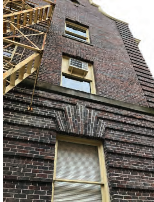
AC units installed in windows, not original.
