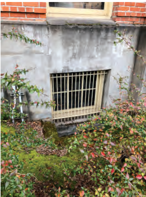
Water damage on window sills; basement windows with bars that are not original.
