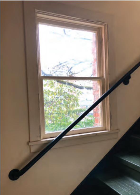
First Floor Stairwell (Railing intersects window)
