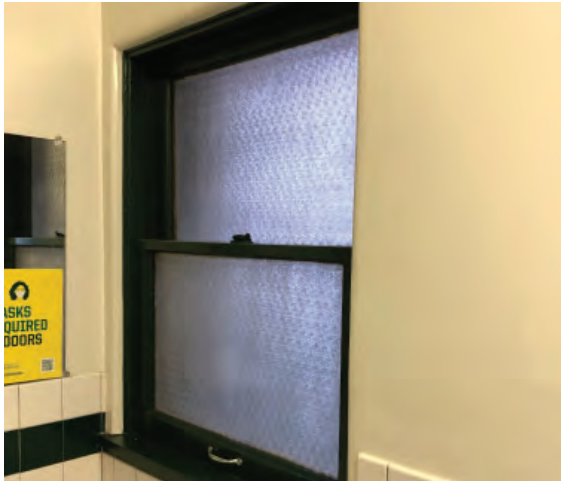
Room 207 Womens Restroom
