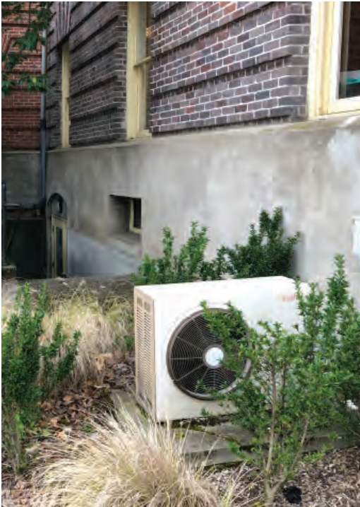
Mechanical systems added to exterior facade in exposed location.
