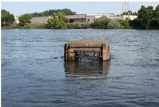
Figure 5 Intake for Alton Baker Park Cano Canal
