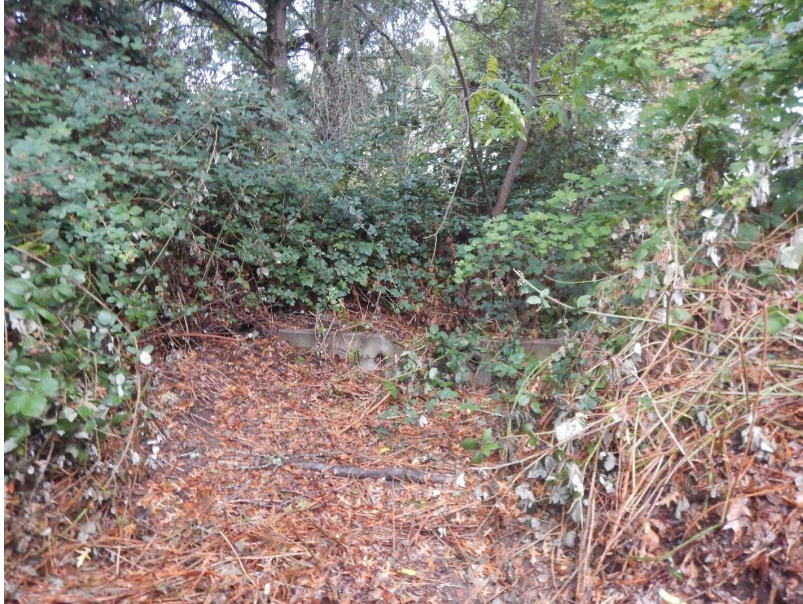
Figure 5. Concrete weir located in bioswale, in need of blackberry removal and re-grading
