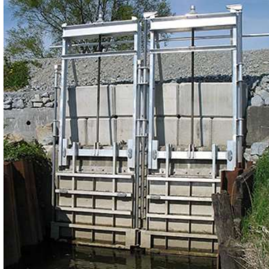
Figure 18. Sluice gate example
